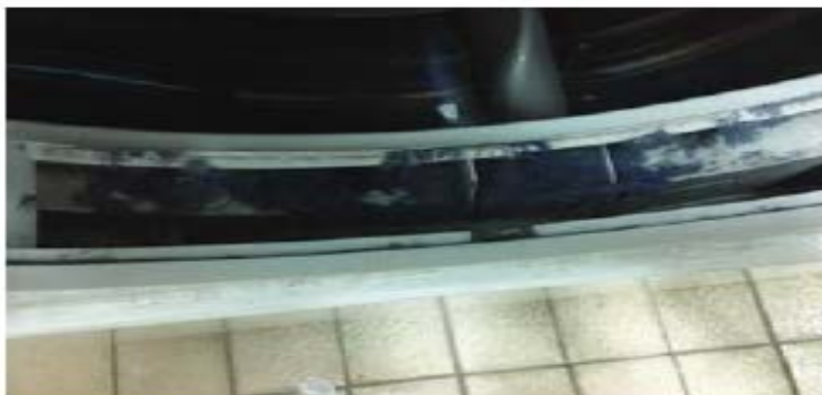
Filter chamber also getting blocked by lint
